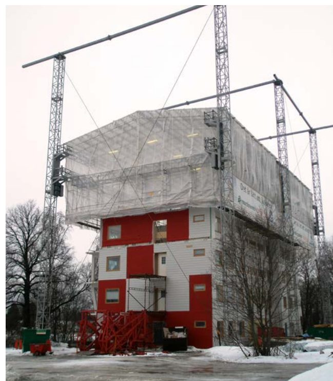
Example of climbing weather protection for dry construction with a high degree of prefabrication.
