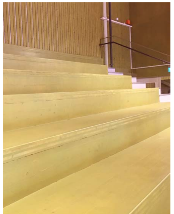
Stepped ledges provide standing room or seating, forming stands in sports venues and halls, Järfälla, Sweden.
