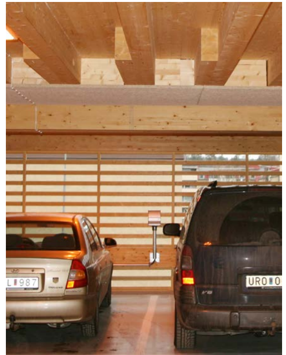
CLT panels combined with glulam beams. Intermediate floor structure in car park, Skellefteå, Sweden.
